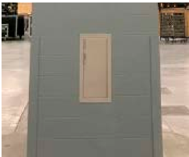
Column with fire extinguisher
